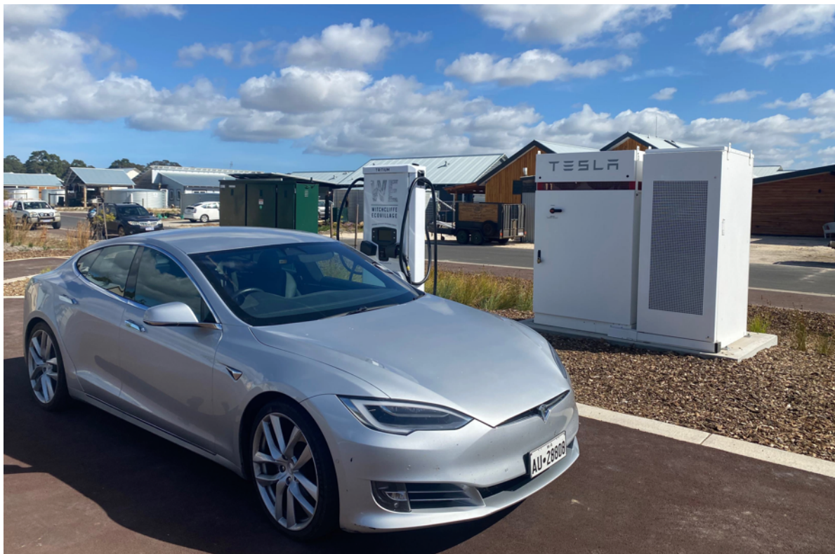
Figure 9. EV in front of Powerpack battery, EV Charger and SMSB in Cluster 1B
