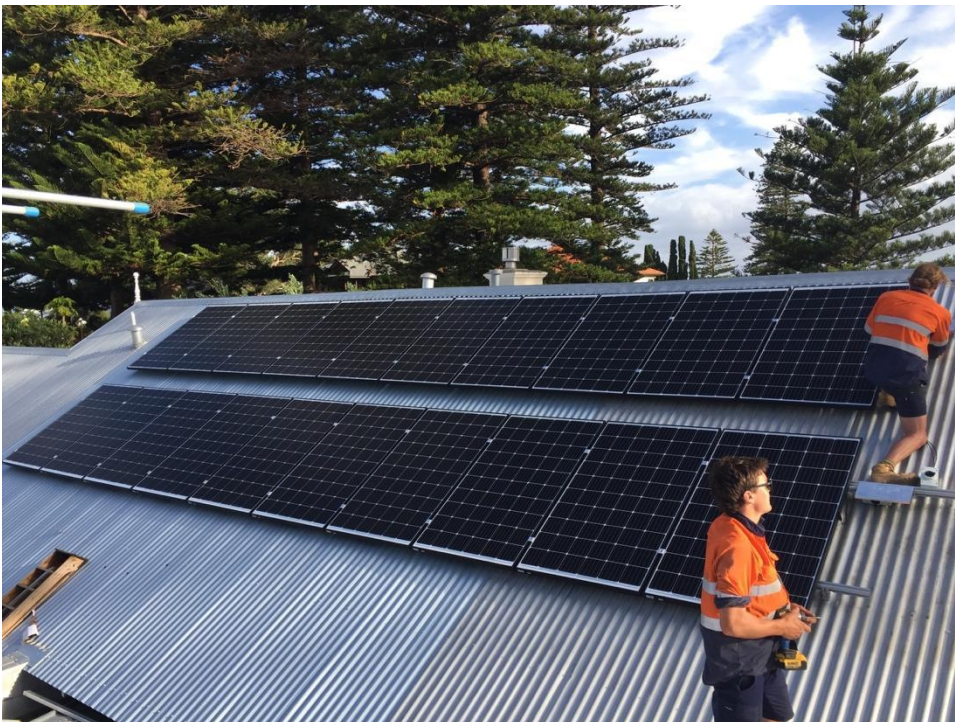
Figure 34. 6.4kW PV array, Cottesloe
