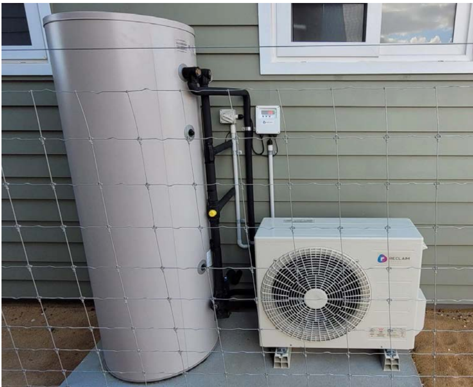
Figure 8. 315L Reclaim system installed in cluster 2B
